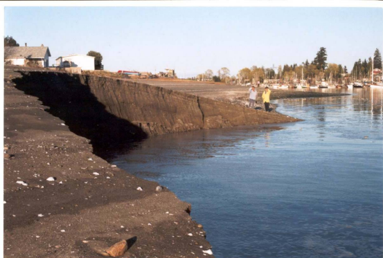
Figure 4. Headwall from collapse of Mapleguard Spit in 1999. Results from a similar event were observed in 1998 as well. (photo compliments P. Monahan)
