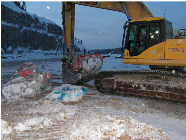
Figure 7. Blocks selected for the in situ rolling rock test The rock fall trajectories were observed as they crossed the road at the base of the cut; the locations of the last two impact points were surveyed. A film recording of each test was made with a digital camera, the high speed camera did not work as these tests were conducted during a cold winter day.
