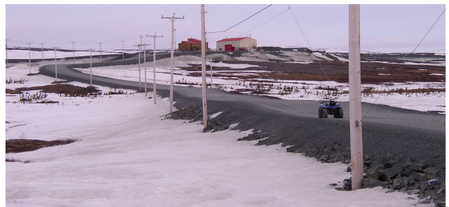
Figure 4: South view of the localized zones of thaw subsidence along the access road to the airport of Umiujaq. The all-terrain vehicle is located in one zone of thaw subsidence. Note the snow accumulation on each side of the road embankment. The photograph was taken in April 30 th 2007. The snow cover was already degrading following the spring warming.
