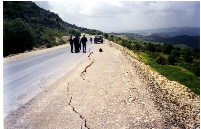
Figure 7. Initial signs of instability, January 2002.
