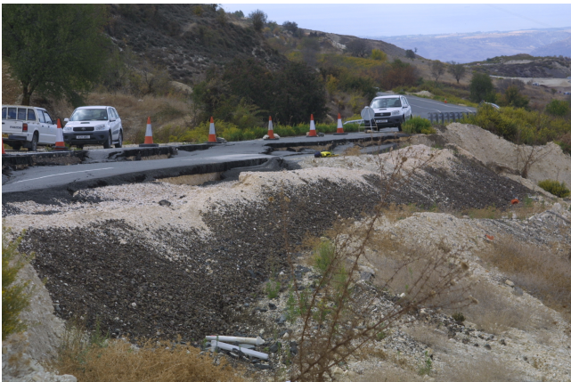
Figure 15. Deterioration of the highway, 2005.
