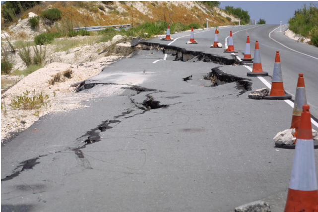
Figure 14. Deterioration of the highway, 2005.
