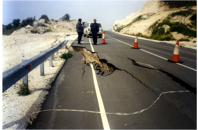
Figure 9. Signs of instability, April 2003.
