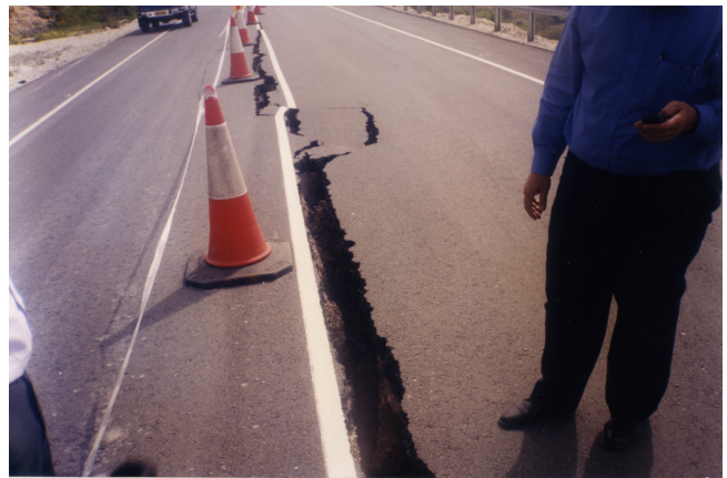
Figure 10. Signs of instability, April 2003.
