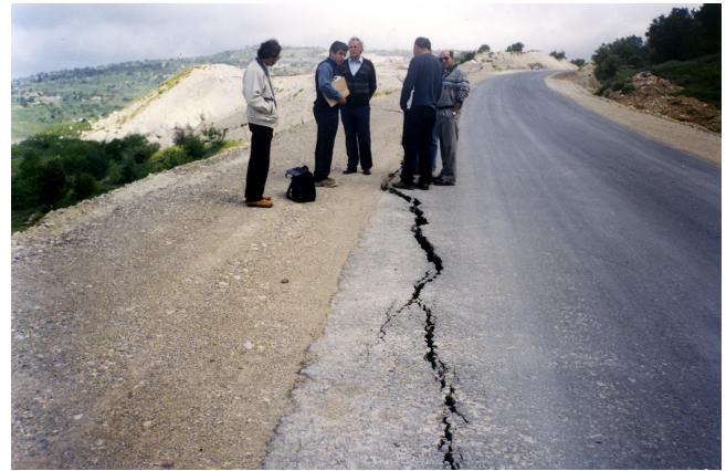
Figure 6. Initial signs of instability, January 2002.
