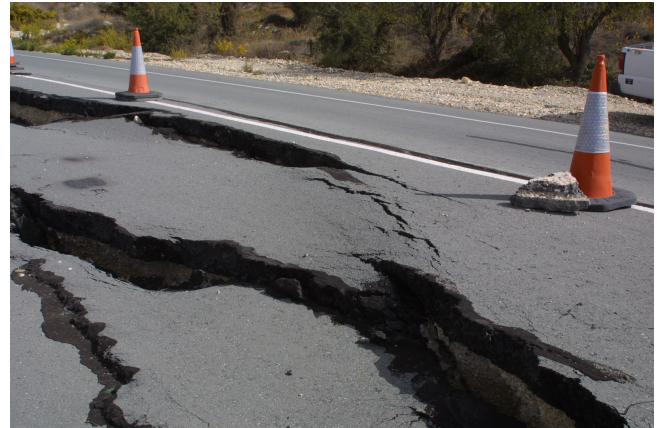
Figure 17. Widening cracks, November 2006.
