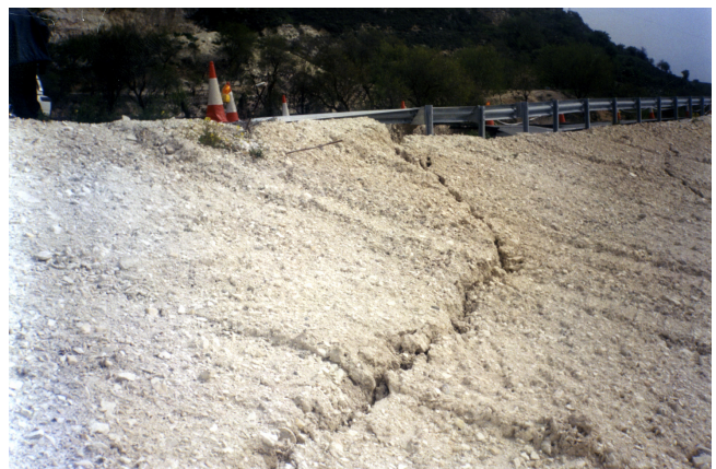
Figure 11. Signs of instability, April 2003.
