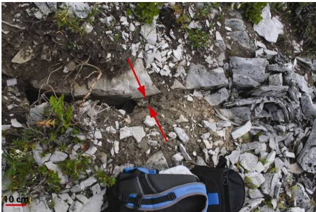
Figure 13: View of the main crack detected under Third Peak. The main opening direction is 060 and the opening is around 15 centimeters.
